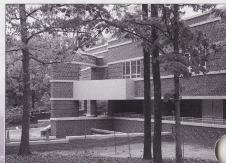
The new Heart and Vascular Center (shown above and below) is expected to be completed by late summer.
