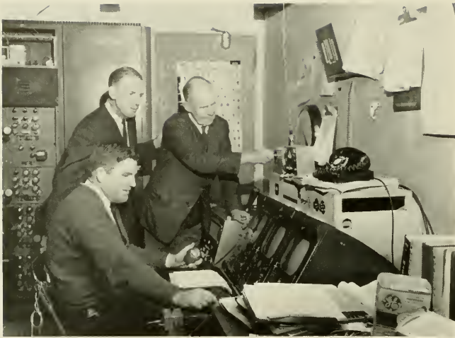
METICULOUS TUNING of equipment insures the engineering crew of a clear telecast.
